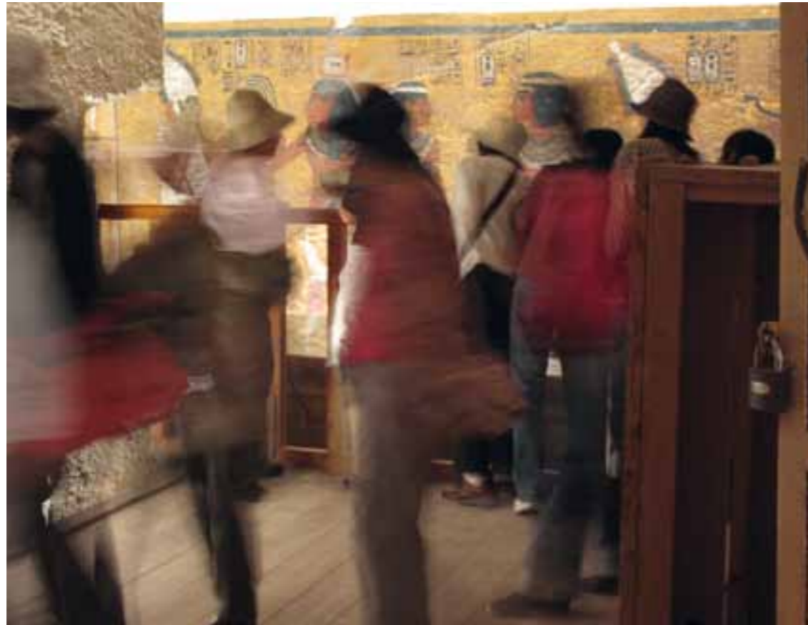
The visitors have a significant impact of the temperature and levels of humidity inside the tomb. This creates a dynamic situation in which the plaster surface is forced to expand and contract. This action will force it to detach from the rock.
