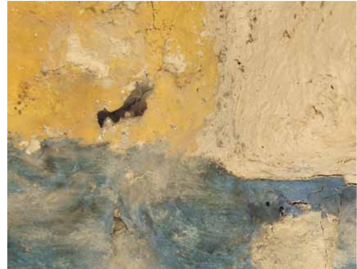
At the top of the north wall the plaster is moving away from the rock to a dangerous degree. Some filling and painting has already been carried out but a large area is in imminent danger of collapse.
